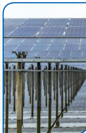
Shouxian Fishery-PV Power Plant 壽縣漁光互補電站
